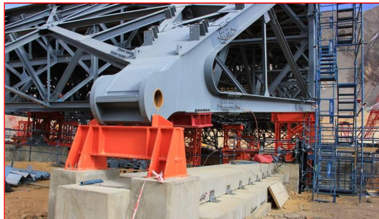
Figure 8. The support at the outside of the side girder. At the concrete skid lane, skid tracks will be installed. The hole is used to make the connection of the roof in its final position with the foundation
