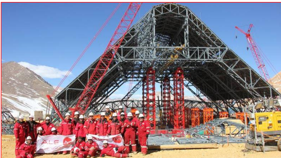
Figure 14. The ALE crew in front of the just jacked up stockpile building roof.
